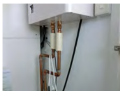
Boiler Thermal sensors
