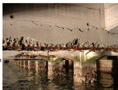
Fig. 2 Example of deterioration (Chloride-induced corrosion)
