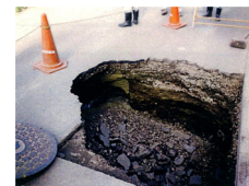
Road cave-in due to corrosion of sewer pipe
