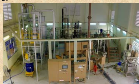
Biomass Facility and Plant in HCMUT
