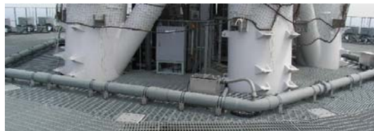
Lightning current observation system installed on 497m point of Tokyo Skytree.
