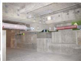
seismic isolation and oil damper
