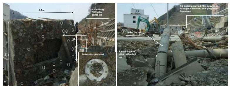
Fig.3 (below) Onagawa town was one of the most seriously tsunami-engulfed towns/cities along the Sanriku coast line. It was shocking that buildings with pre-stressed high-strength concrete piles were uprooted at several locations in Onagawa, all the more pile-supported RC and/or steel-frame structures had been considered to be possibly good for tsunami shelters.
