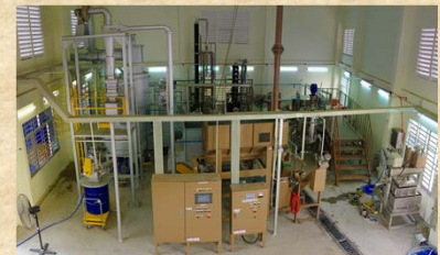
Biomass Facility and Plant in HCMUT
