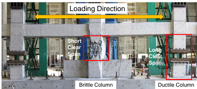
Damage after IDR=1/33rad.
