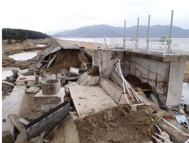
Coastal levee damaged by tsunami. (Ishinomaki city)
