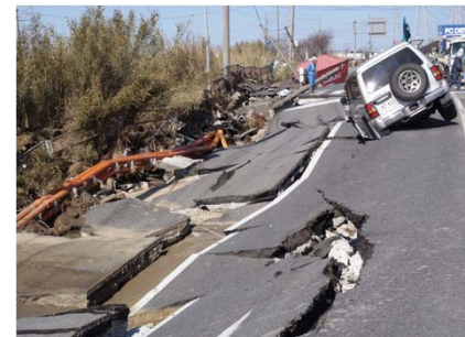
Road damaged by liquefaction followed by tsunami attack (Kamisu city)
