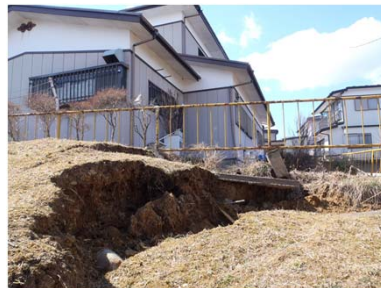
Damage of artificial earth fill for housing estate. (Sendai city)
