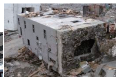
Building flushed away by tsunami
