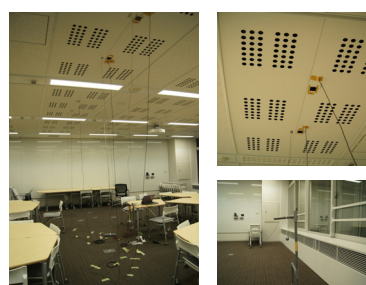
■ Field measurements of the performance of a radiant ceiling system
