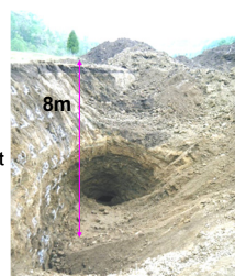
Soil pipe found at the location of cave-in
